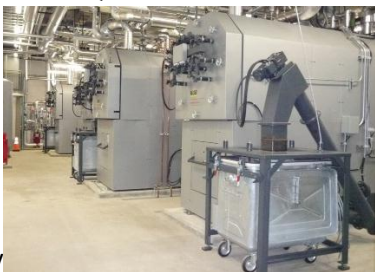
Figure 12 — Bouilloire Pyrotec aux granules de bois
