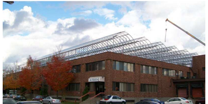
The Lufa Greenhouse under construction. It will be completed by the end of 2010. Seeding will begin in late January and full harvests are expected by early April.
