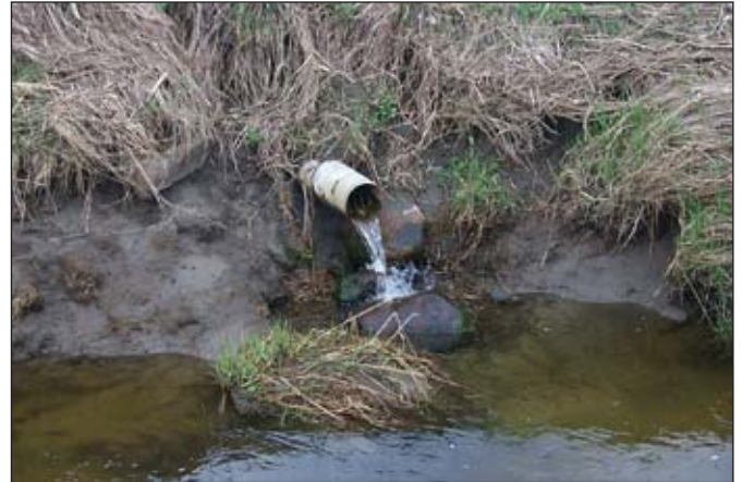
Photo 12: Erosion at a drain outlet Source: Mikael Guillou, MAPAQ
