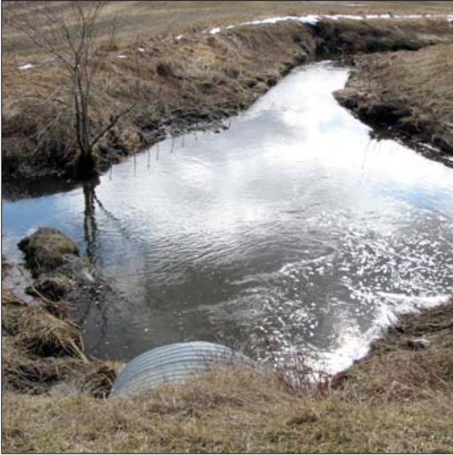
Photo 8: Widening of the streambed downstream of a culvert Source: Mikael Guillou, MAPAQ
